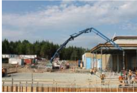
Fig. 1: FRP-reinforced concrete tank, Qc, Canada.
